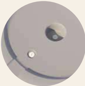
OVERFLOW HOLE AND RESERVOIR DRAIN HOLE
